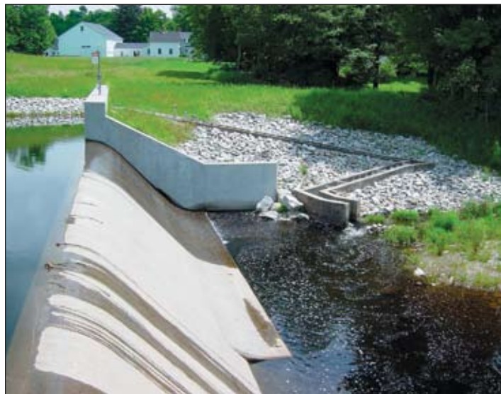
Crest of Highland Lake Dam and fishway with sediment bar obstructing attraction flow at fishway entrance. These improvements will help to restore runs of river herring and American eel.
