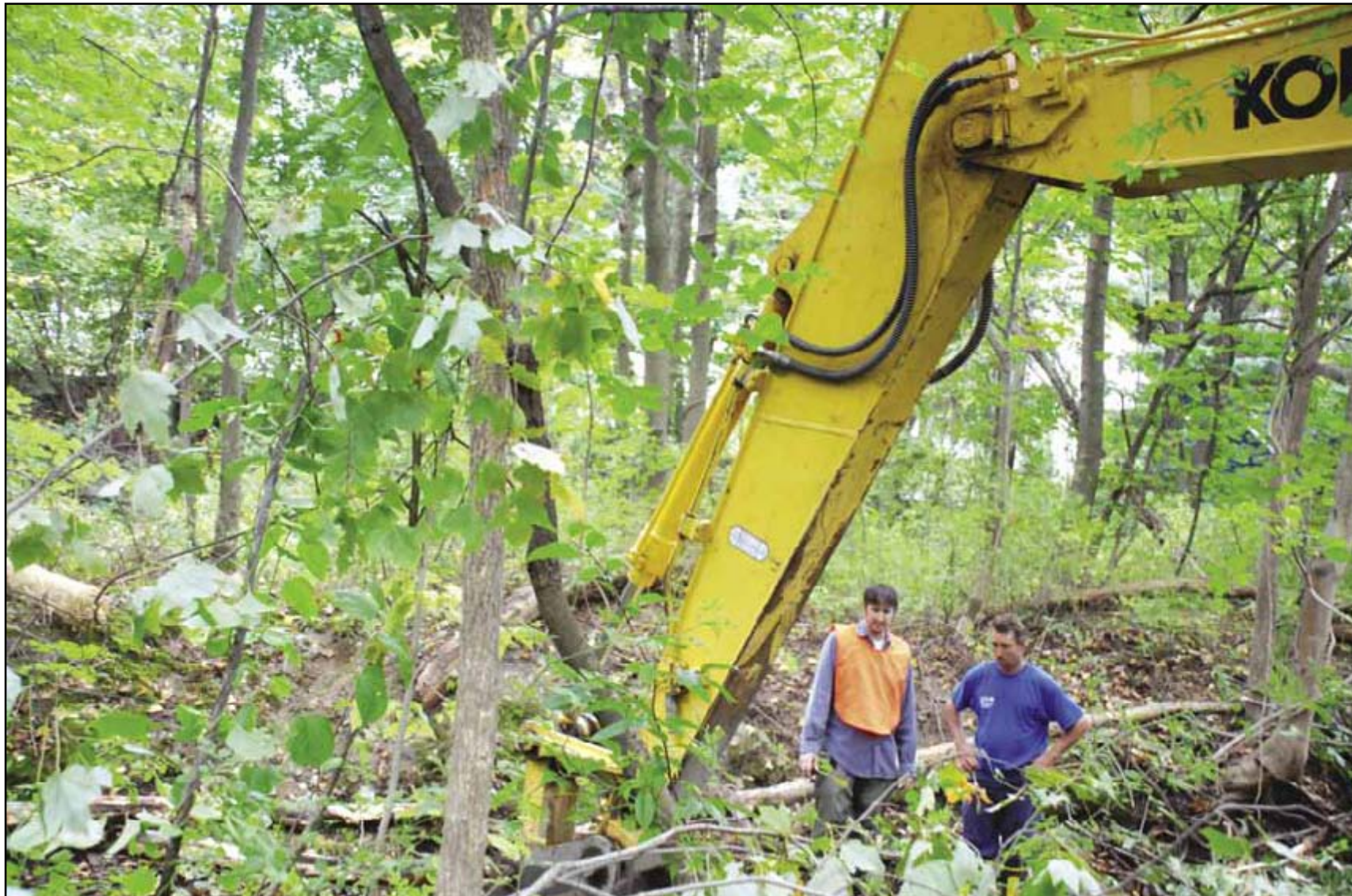
Workers from the city of South Portland and volunteers breached a manmade berm along the bank of Trout Brook on Friday, Sept. 28 to allow the brook to access a floodplain when storms cause the water levels to rise. The work is part of what Fred Dillon of Water Resources Protection called a "modest but meaningful" project to restore the water quality of Trout Brook. (Marc Filippino photo)
