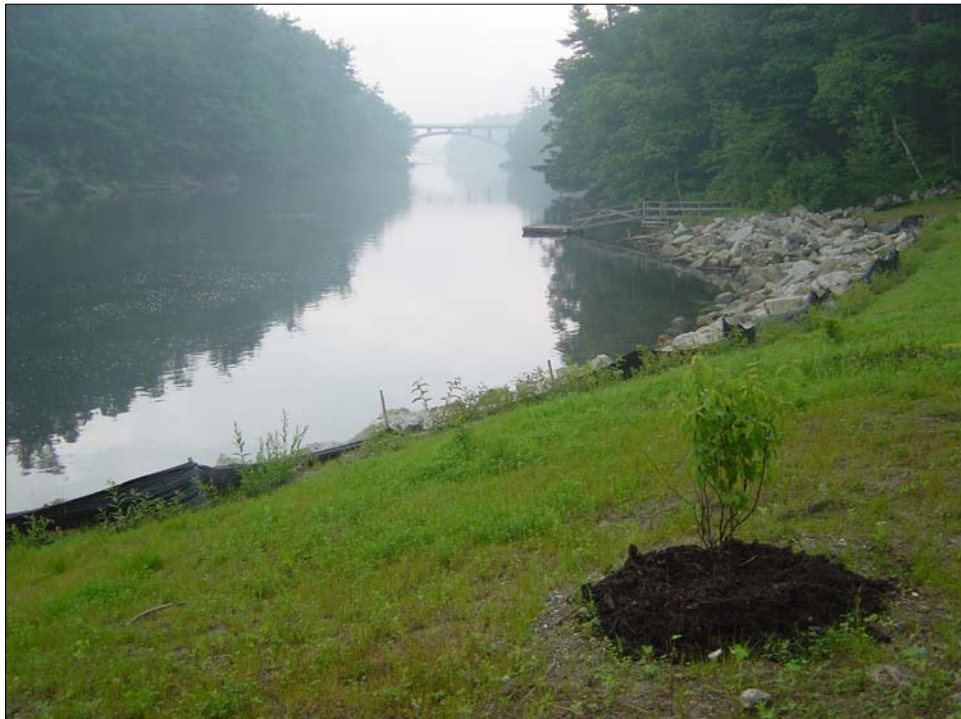
June 2006. Presumpscot River southern shore facing downstream at site of Smelt Hill dam removal. Note willow waddles planted during fall 2005 flourishing in front of silt fence along the length of the site.
