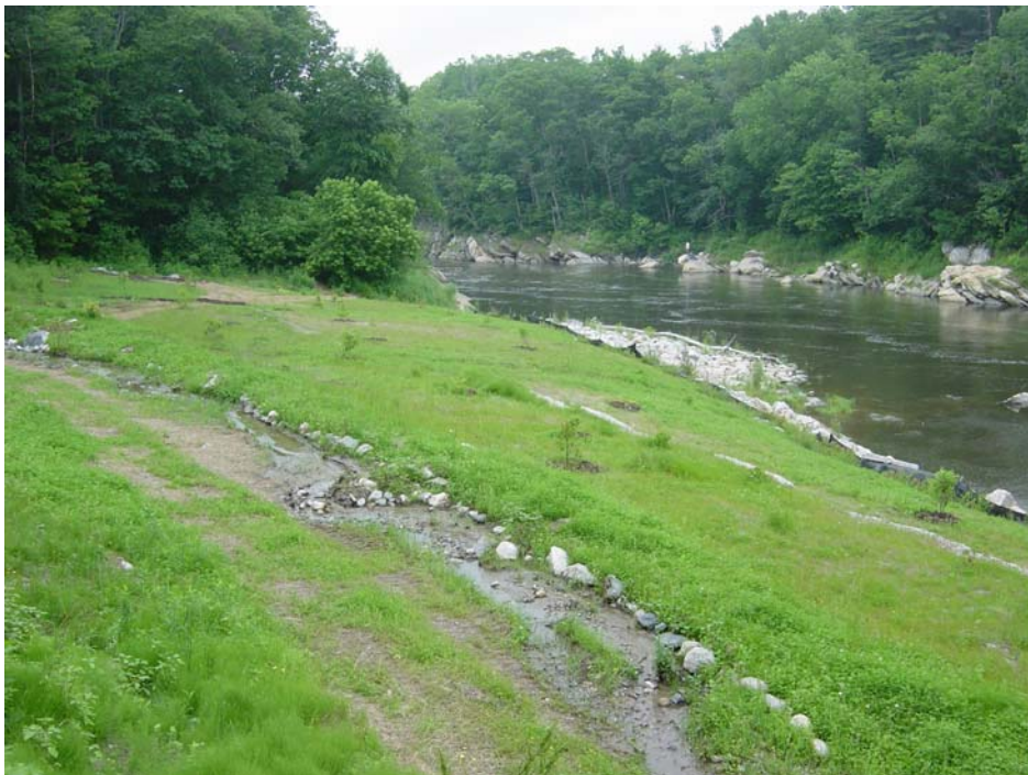
June 29, 2006. Site post- Phase II implementation. Note granite wall to the left, which was unearthed during Phase I regrading activities.
