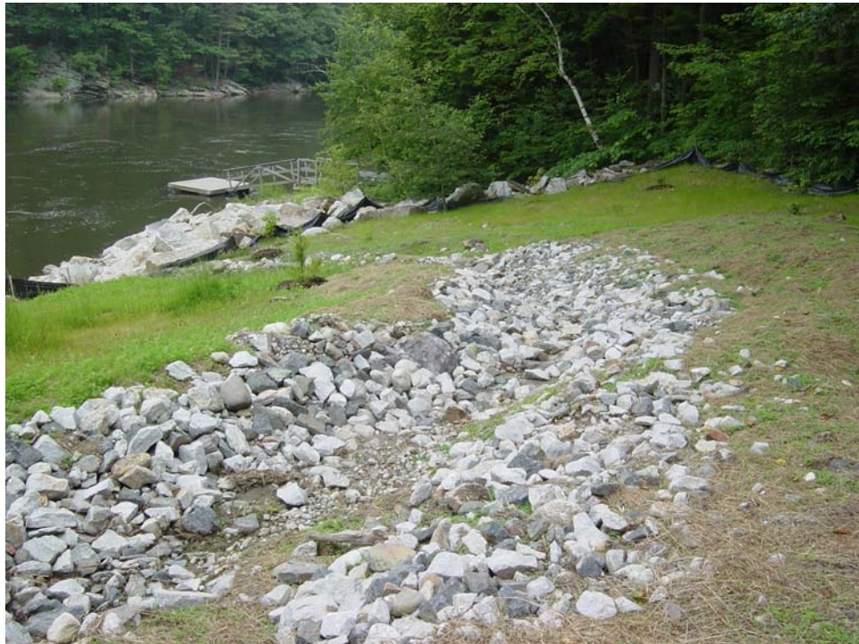
June 29, 2006. Smelt Hill swale, lower run, post Phase II adaptive management implementation.
