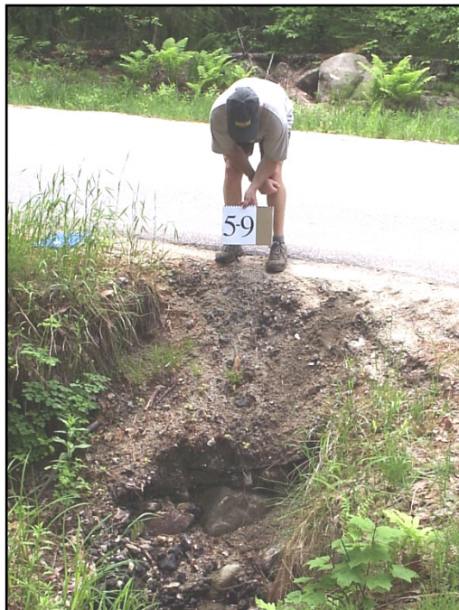
A Pleasant River Watershed Survey volunteer documents road shoulder erosion above a culvert washing into a tributary of the Pleasant River.
