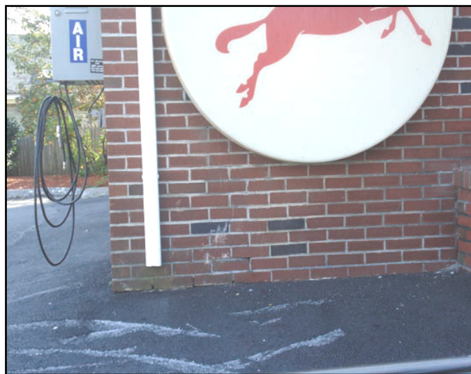
Downspouts draining onto impervious surfaces rather than being filtered into the ground are considered potential "hotspots" due to the potential pollutants the stormwater can pick up and wash into the Pleasant River.
