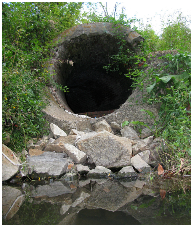
Combined sewer overflow at Capisic Brook in Portland.
