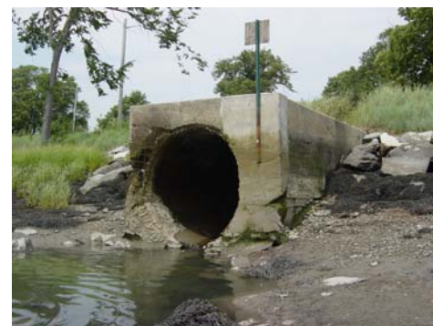
Combined sewer overflows (CSOs) discharge a mix of stormwater and untreated sewage during wet weather. The CSO outfall pictured above empties into Portland's Back Cove.
