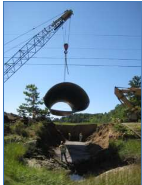
The Adams Road culvert at Thomas Bay Marsh was replaced in August 2011.
