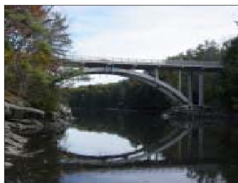
The Allen Avenue Extension Bridge spans the Presumpscot River in Falmouth, Maine.
